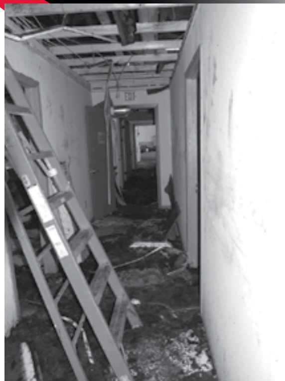
A fire caused by a lightning strike, during one of the many severe storms that hit the Wisconsin Dells area in June, caused significant damage to one of the buildings at Camp Wawbeek.
